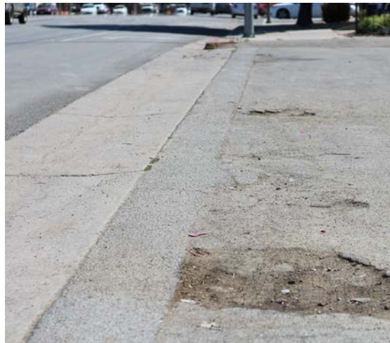
Sidewalks in commercial areas are frequently interrupted by long driveways.
